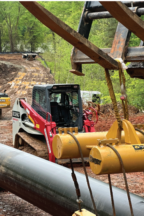
Pull back of 1,305 lf of 30-in. HDPE pipe in a hard rock formation under the Catawba River.
